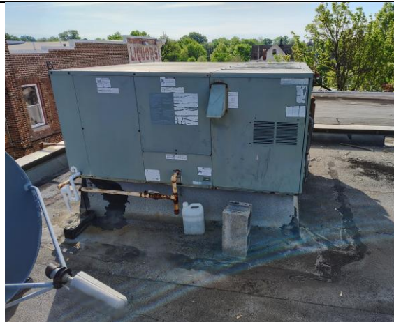
Rooftop Air-Condensing Unit Assumed ODS-Containing Equipment
