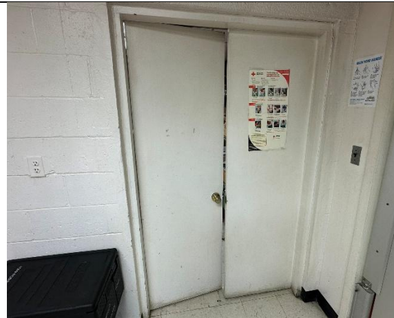
Readings #52 & 53 - White Door and Door Frame Lead-Based Paint
