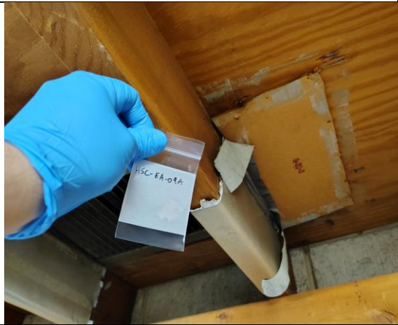
Gray Paper Wrap on Ceiling Joist ACM – 50% Chrysotile
