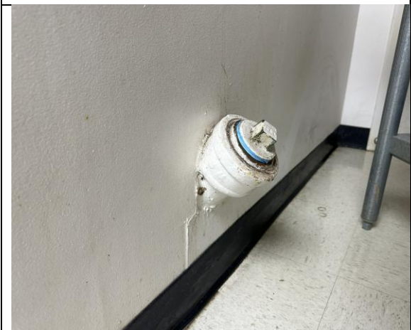
Reading #59 - White Pipe Lead-Based Paint
