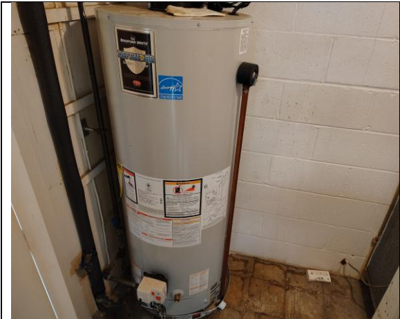
Overview of Room 25 Kitchen Mechanical Room
