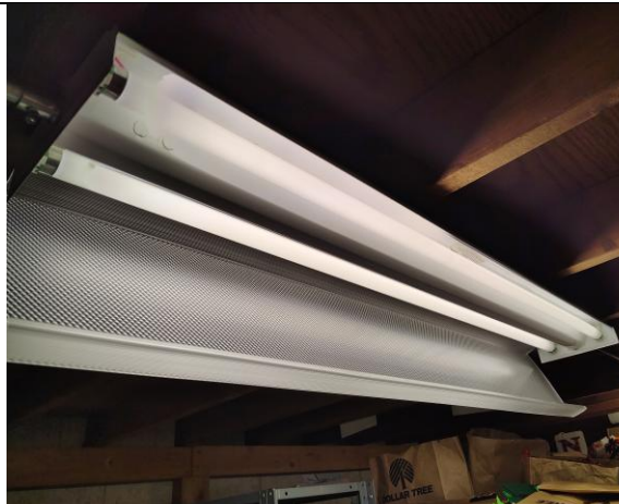
Fluorescent Light Ballast Assumed PCB-Containing Equipment
