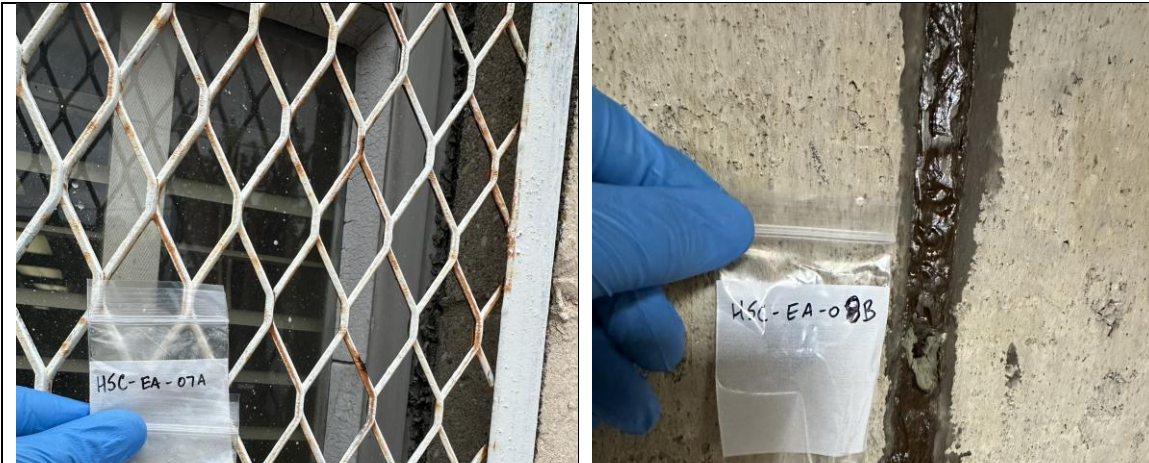
White Window Glazing ACM – 2% Chrysotile
