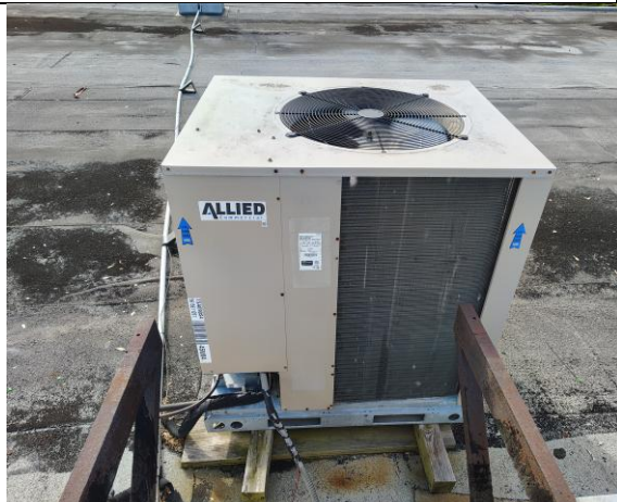
Representative Rooftop Air-Conditioning Unit ODS- Containing Equipment
