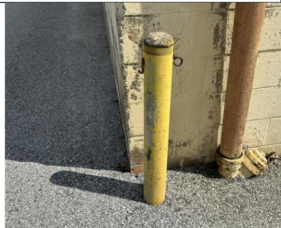
Reading #195 - Yellow Parking Bollard Lead-Based Paint
