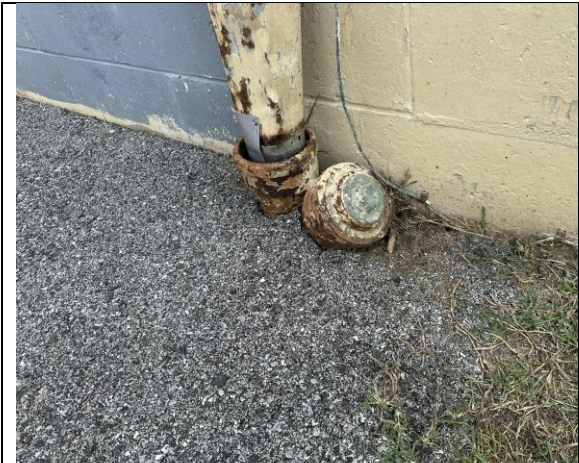
Reading #191 - Exterior Pipe Lead-Based Paint
