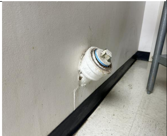
Reading #59 - White Pipe Lead-Based Paint
