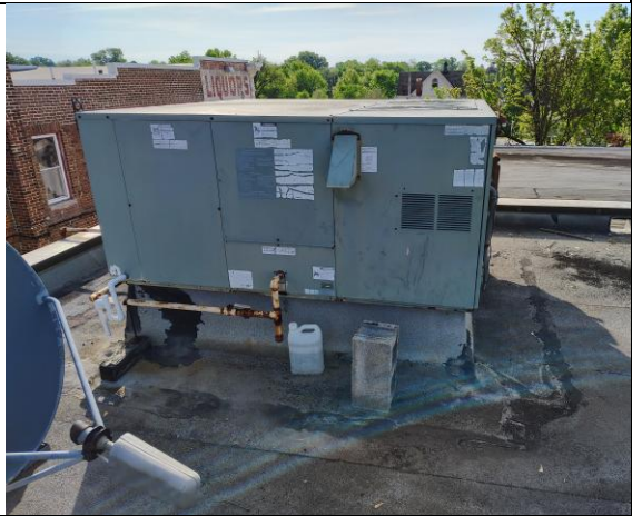
Rooftop Air-Condensing Unit Assumed ODS-Containing Equipment
