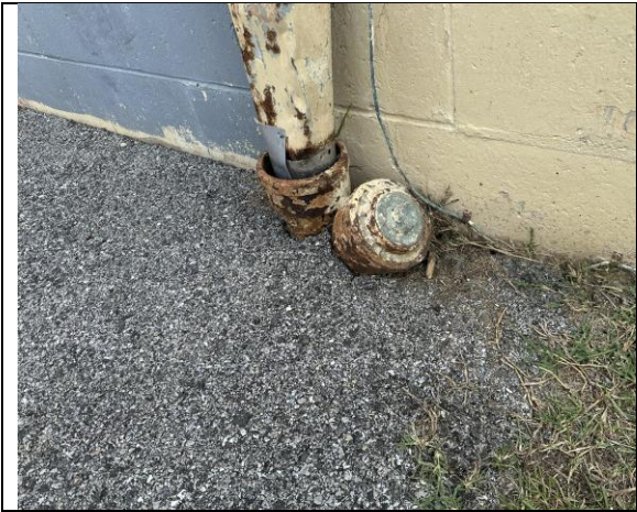
Reading #191 - Exterior Pipe Lead-Based Paint
