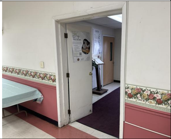
Reading #27 - White Door Frame Lead Based Paint
