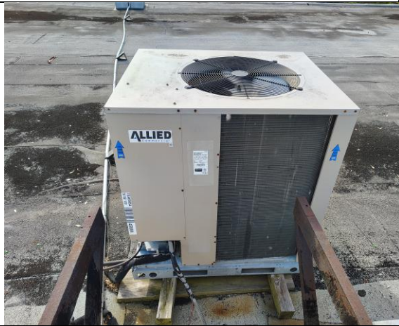
Representative Rooftop Air-Conditioning Unit ODS- Containing Equipment
