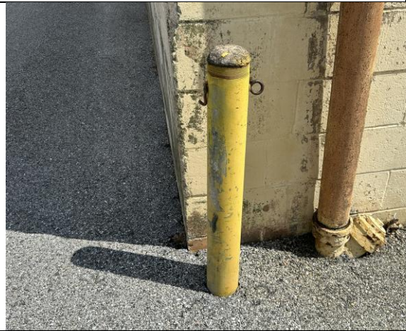
Reading #195 - Yellow Parking Bollard Lead-Based Paint
